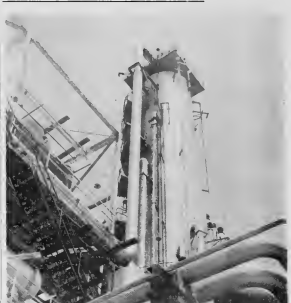
REVAMPED No. 10 Viscosity Breaker (above) went on stream July 21 following renovation after 25 years of service.
